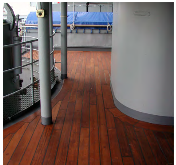
This is the O-3 level starboard signal bridge after similar repairs were made in 2007, it's hard work, but the results are impressive!
