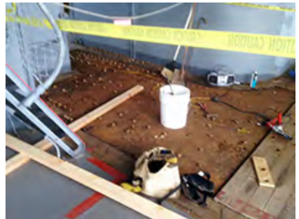
Photo showing work that has just begun on the O-3 level portside signal bridge
