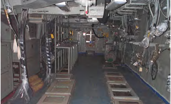
View of the Transmitter Room, January 2001
